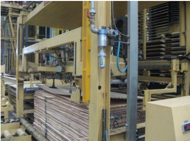
▲ Veneer sheet transfer line in wooden industry
